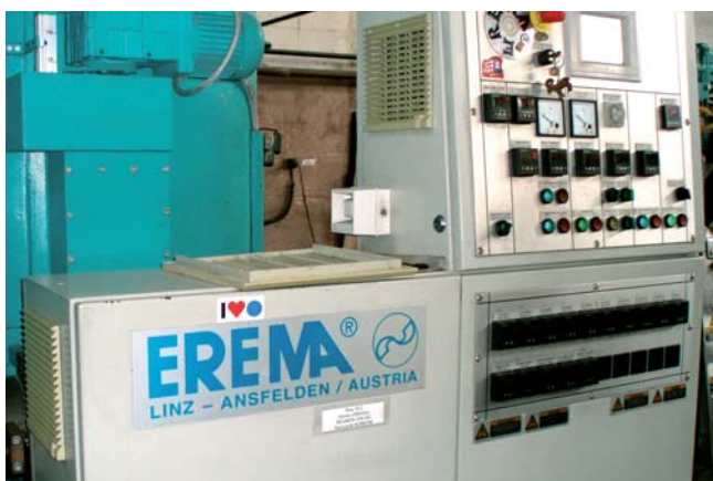
Switch cabinet from Erema with Siemens control
